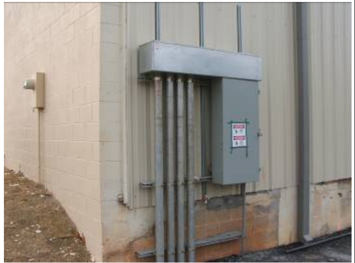
PHOTOGRAPH 14 Recently installed electrical service
