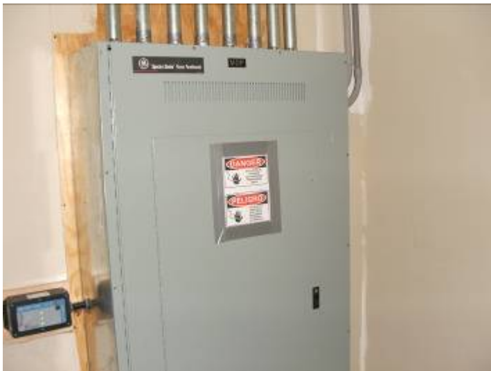
PHOTOGRAPH 15 Main electrical panel
