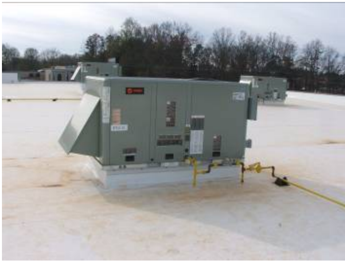
PHOTOGRAPH 13 Recently installed Trane brand roof mounted HVAC unit
