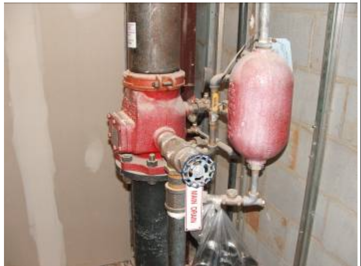
PHOTOGRAPH 16 Fire suppression equipment
